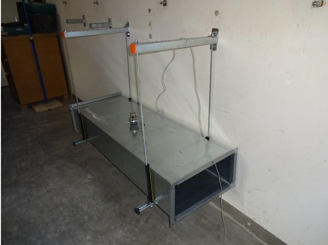
Fig. 3: Ventilation duct, placed on MPC system rails (38/40/2.0) with DÄMMGULAST® rail profiles
