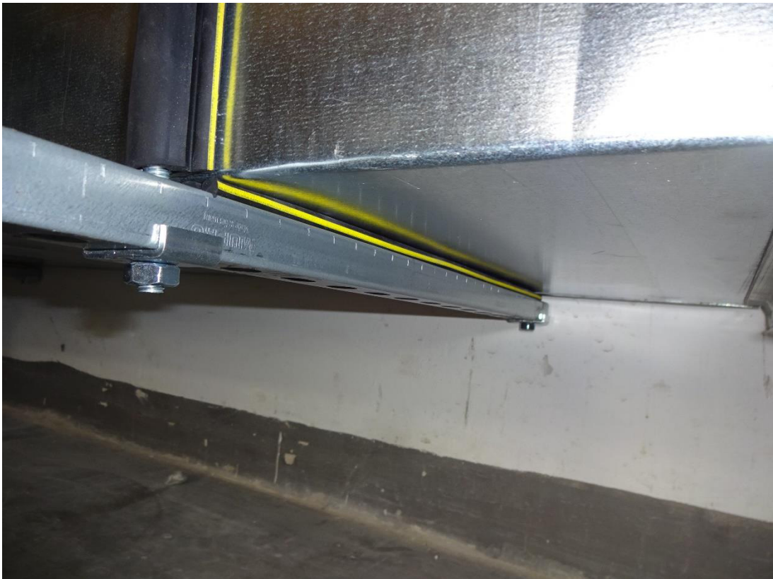
Fig. 4: Ventilation duct, placed on MPC system rails (38/40/2.0) with DÄMMGULAST® rail profiles
